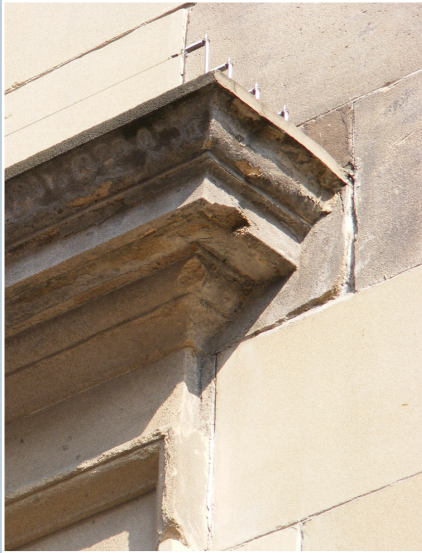
Discreet sprung wires are attached to the top surface of this cornice to deter birds. Miller Street, Glasgow.
