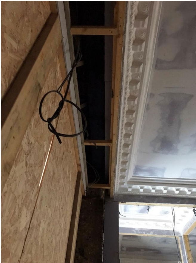
Figure 6 Unsealed gaps at the edge of the separating floor (from within the restaurant)
